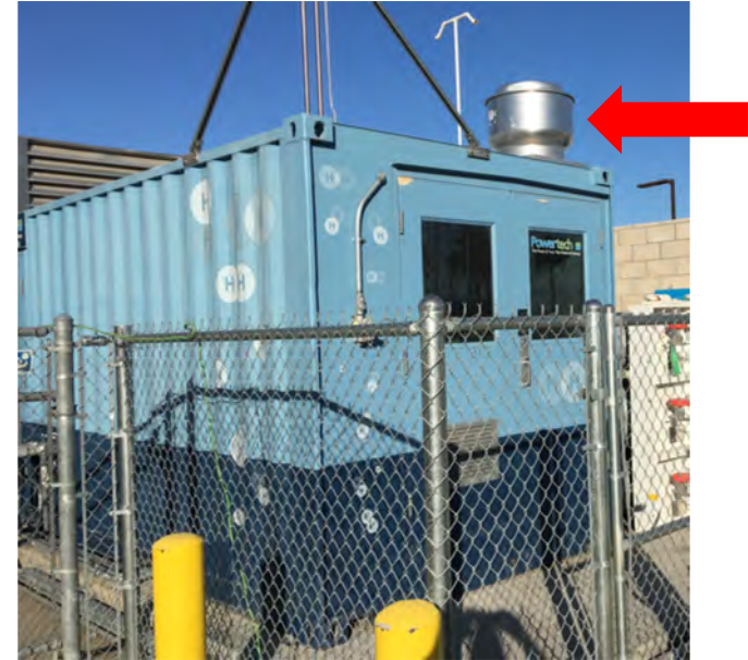
Compressor HEE with mechanical ventilation
