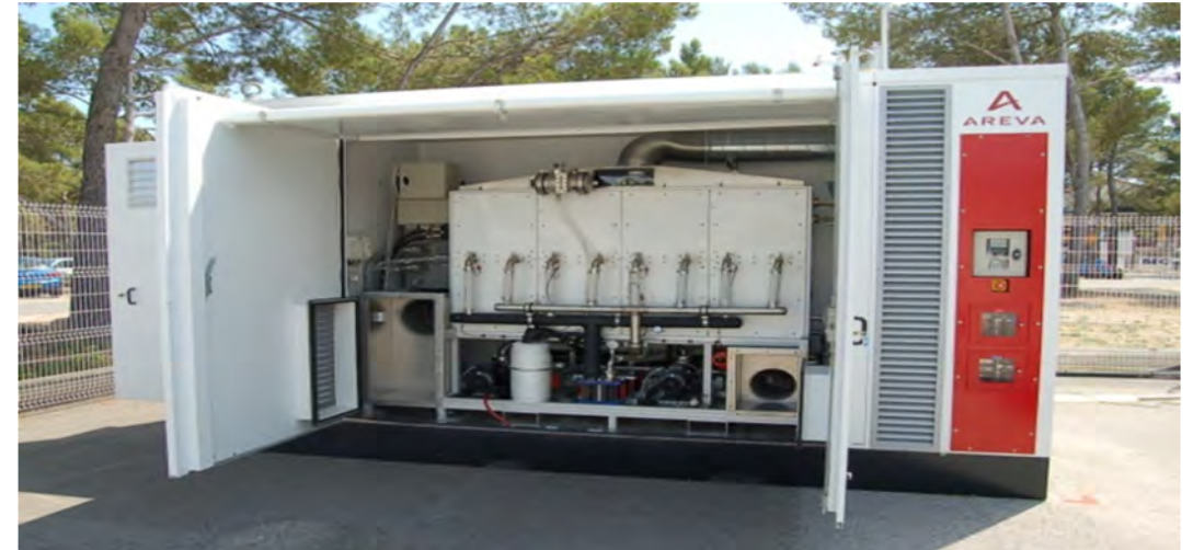
Fuel cell backup power connected to a data center
